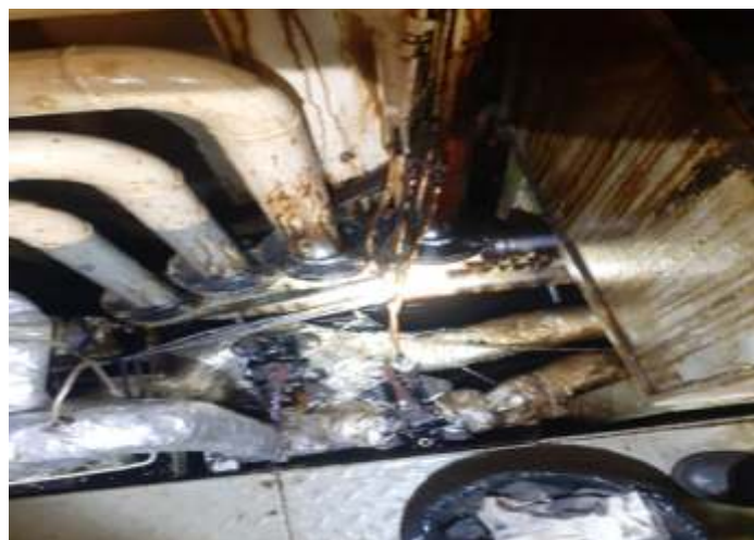
PICTURES OF DEFICIENCIES IDENTIFIED
