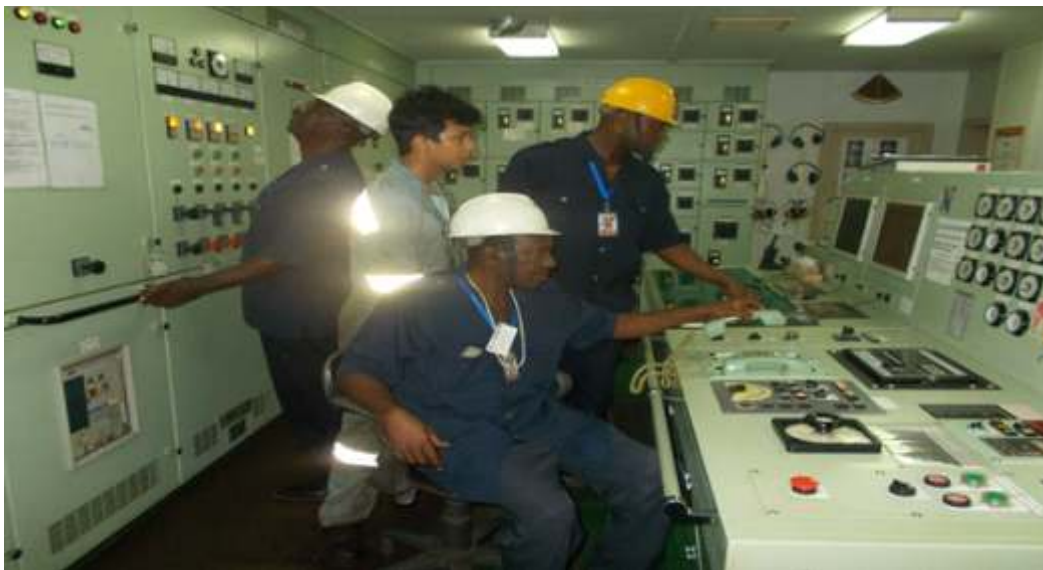
GUINEA PSCOS INSPECTING THE ENGINE CONTROL ROOM
