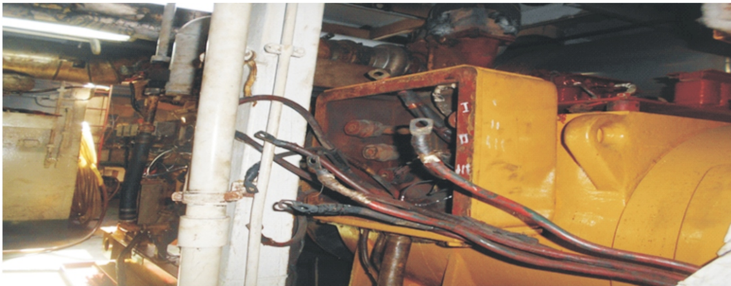
Unprotected electrical cables
