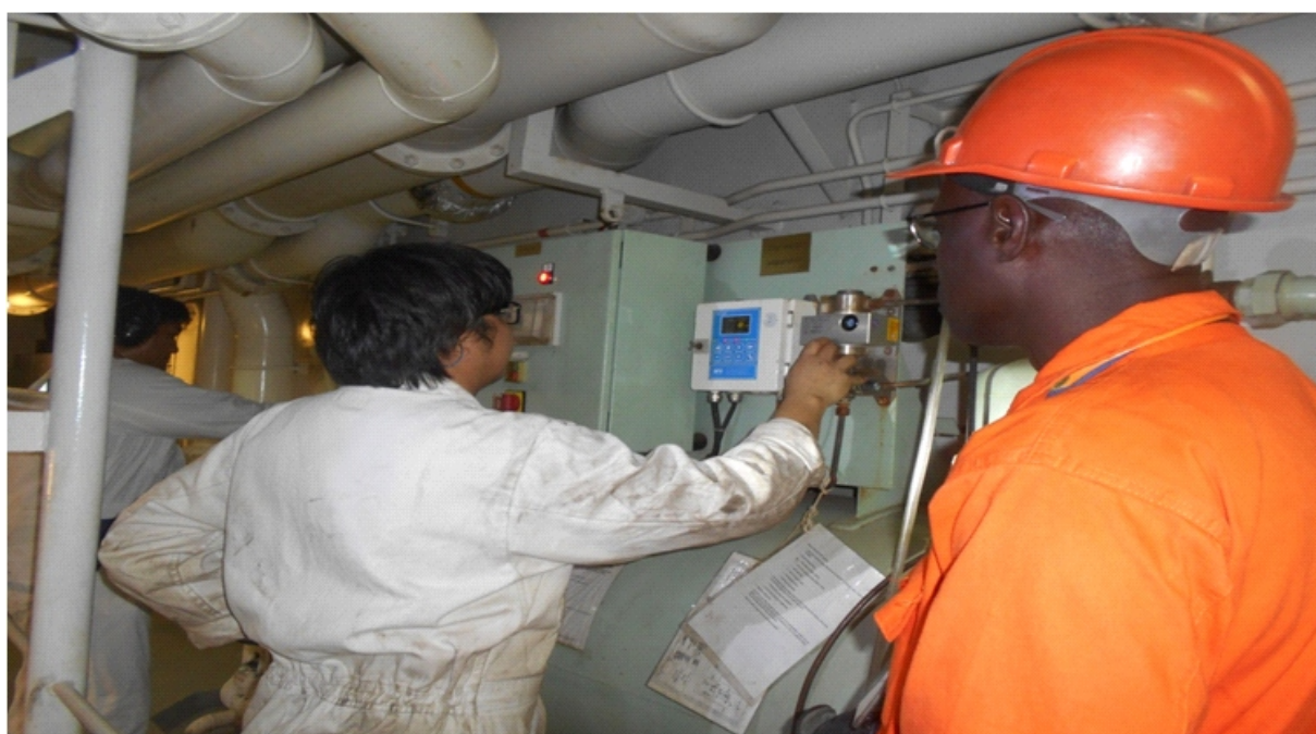
Inspecting pneumatic system
