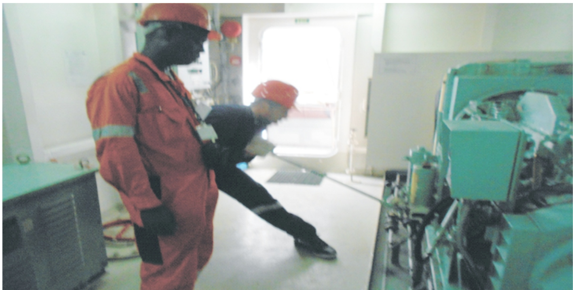
Inspecting Emergency generator
