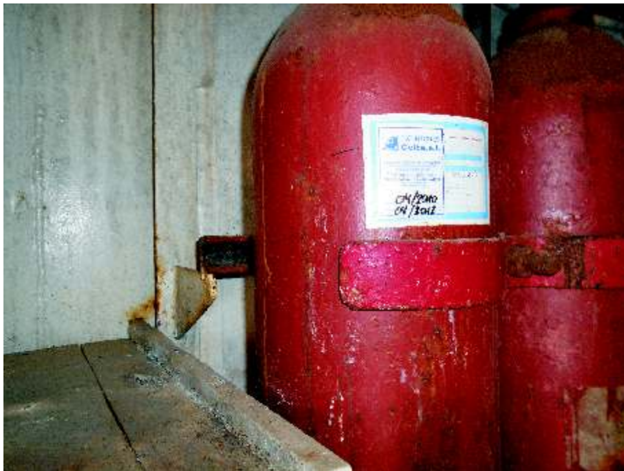
Expired Date on inspection carried out in 2014.
