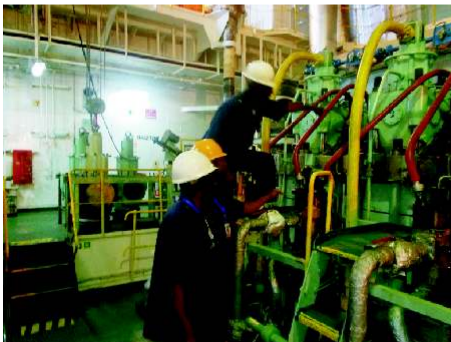
Guinea PSCOs Inspecting the Engine Room.
