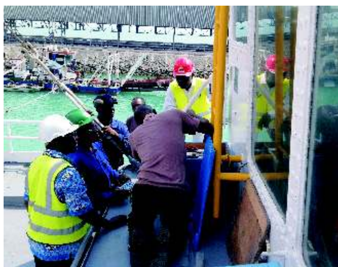
Ghana PSCOs inspecting the Battery Bank
