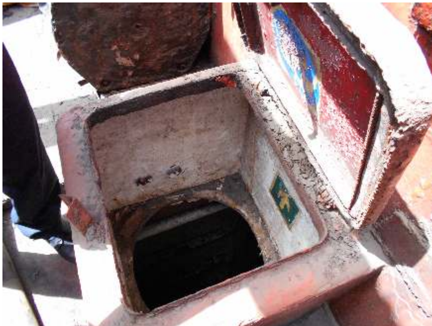
Corroded and Wasted Water Tight Rubber Seal and Support (Water Tight Integrity Lost).
