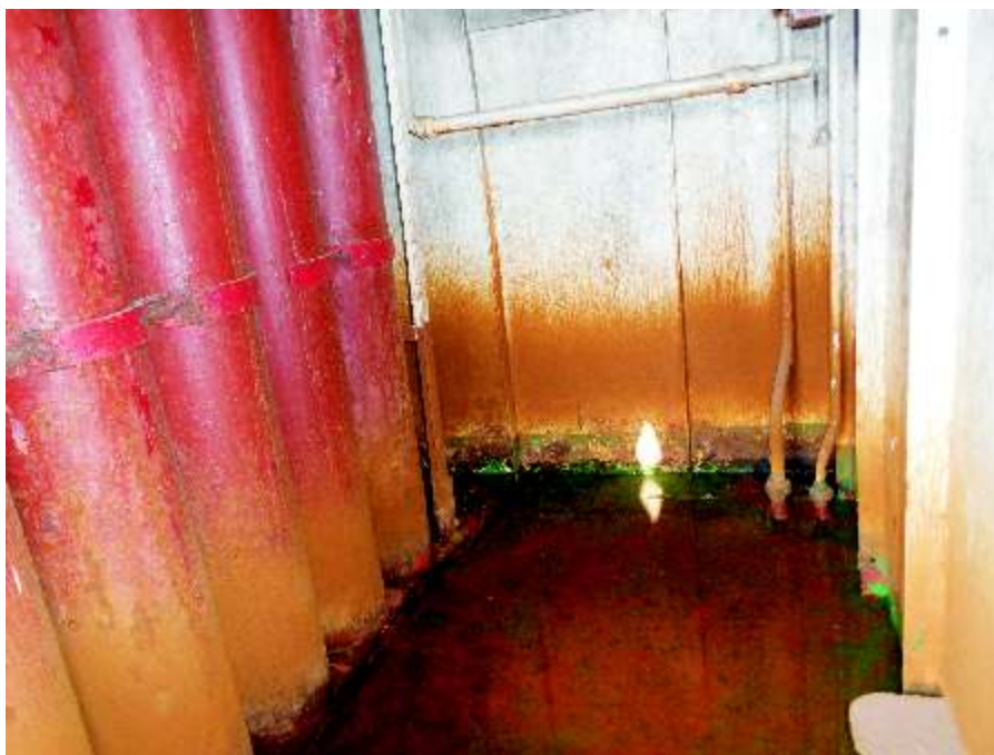
Rusted and Holed Bulkhead allowing Water Ingress into CO 2 Room.
