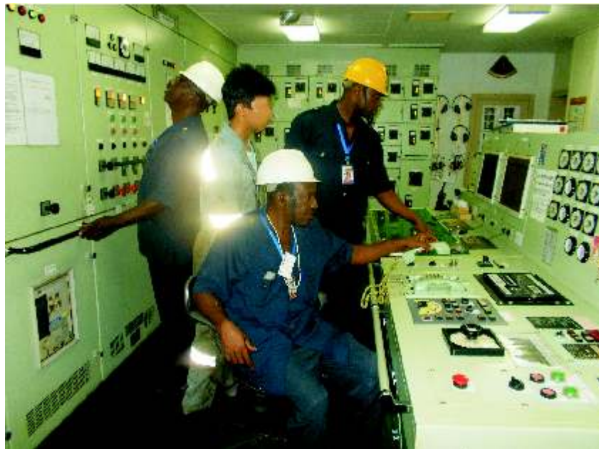
Guinea PSCOs in ER Control Room.
