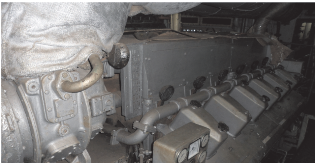
Exposed Exhaust gas pipe on diesel engine
