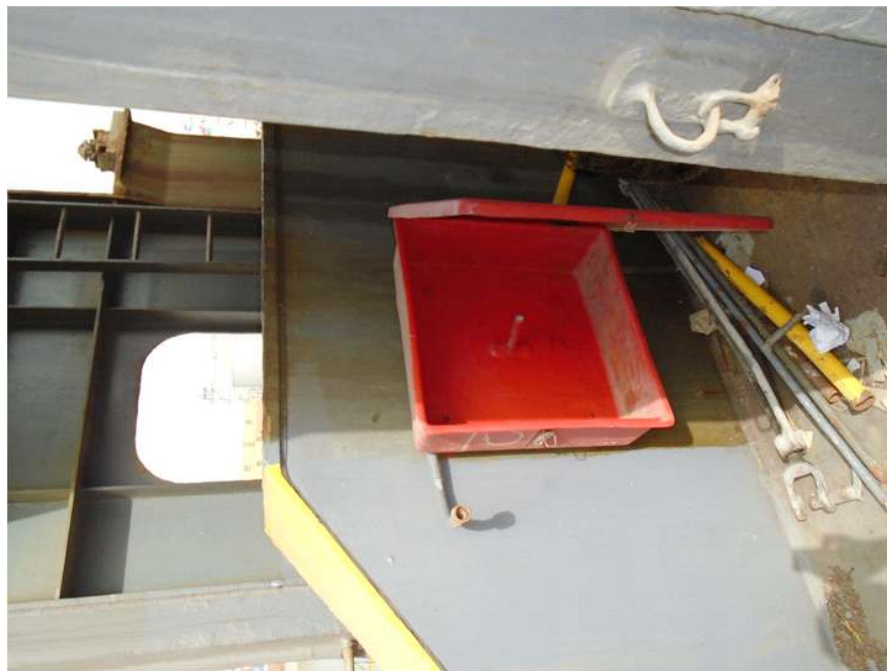
Wasted shackles and empty fire hose box
