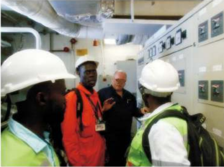
PSCOs inspecting emergency generator switchboard
