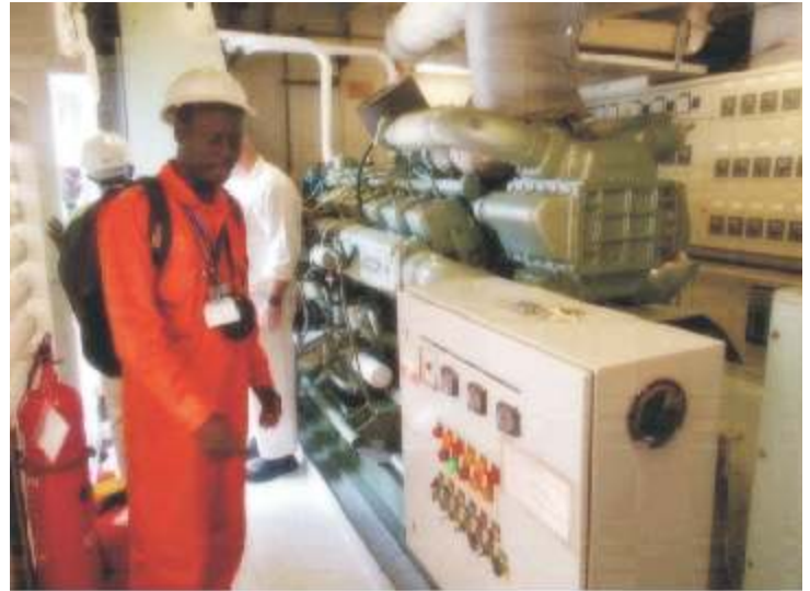
Emergency Generator operation
