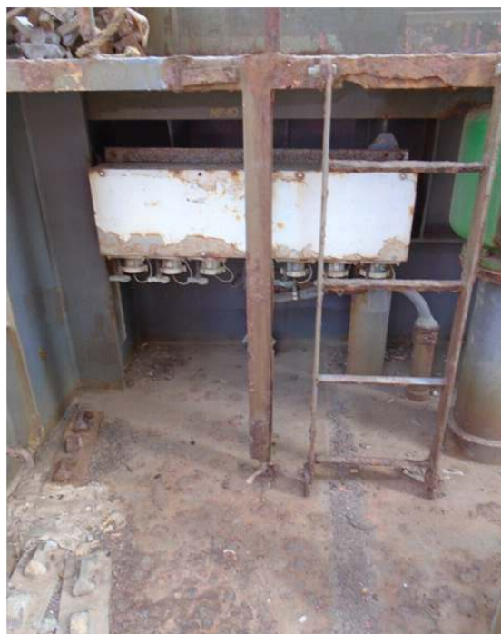
Corroded/ wasted hatch coaming and vertical ladder
