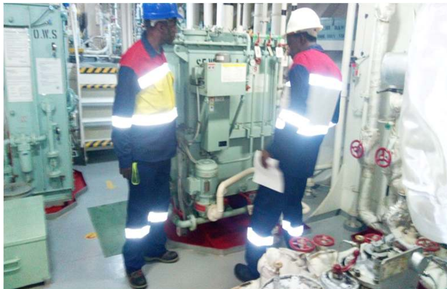
PSCOs by Oily Water Separator and Sewage Plant
