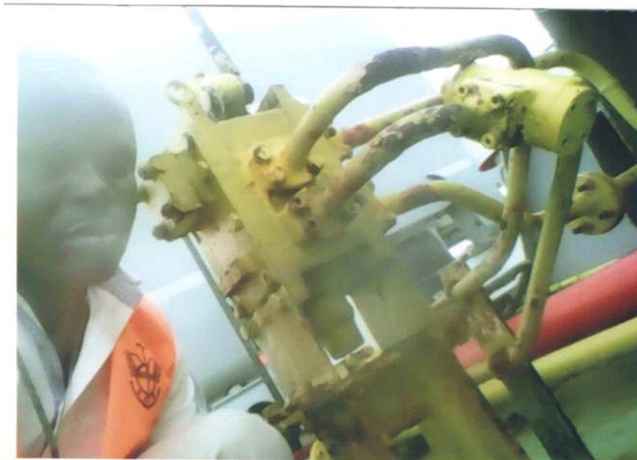
Corroded and leaking hydraulic pipe
