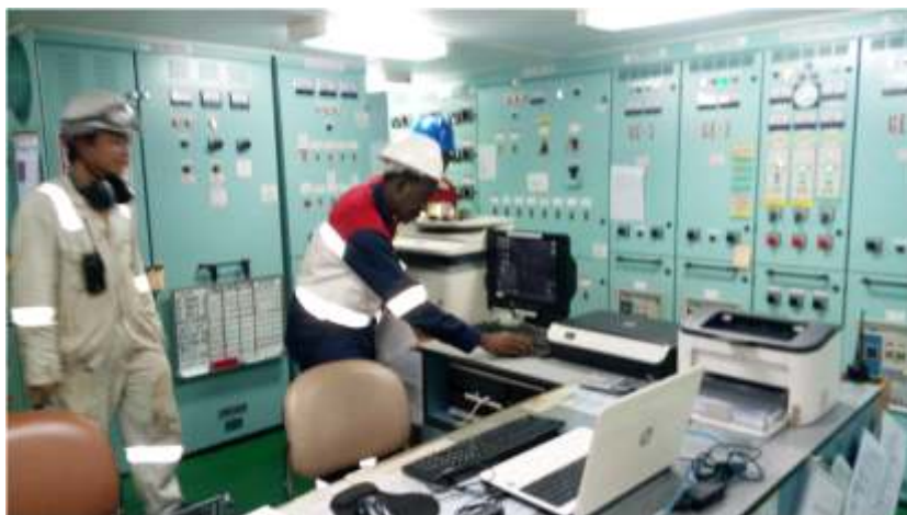
PSCO in E/R control room
