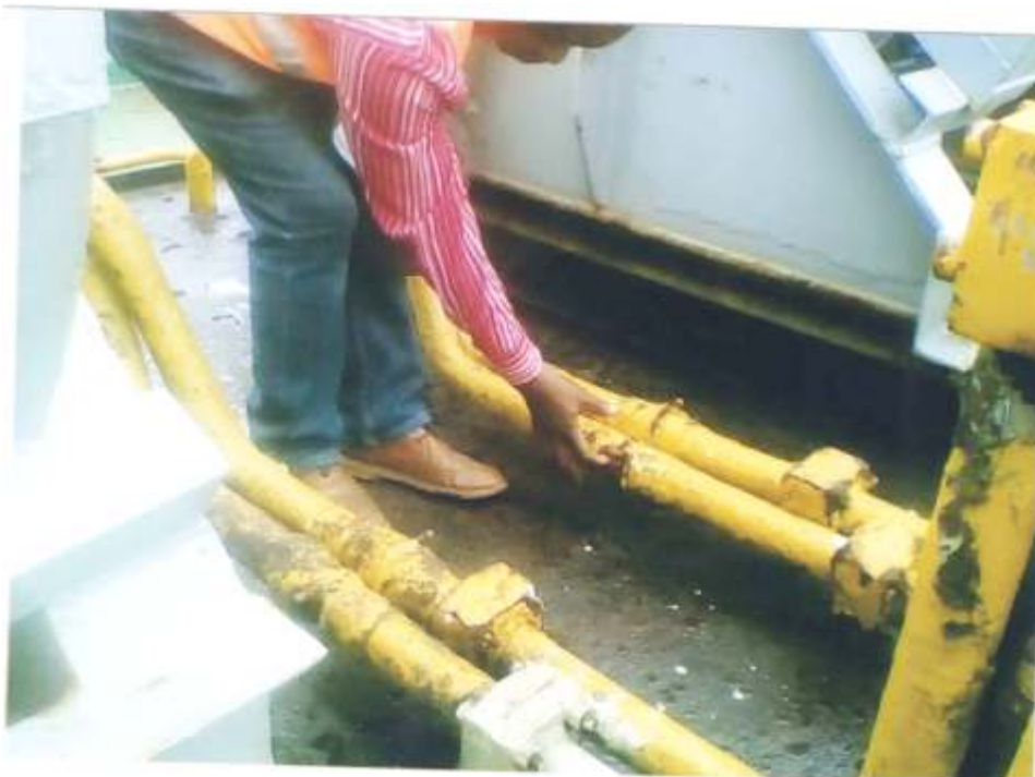
Wasted pipes on deck
