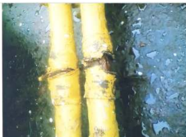
Wasted electric cable conduit
