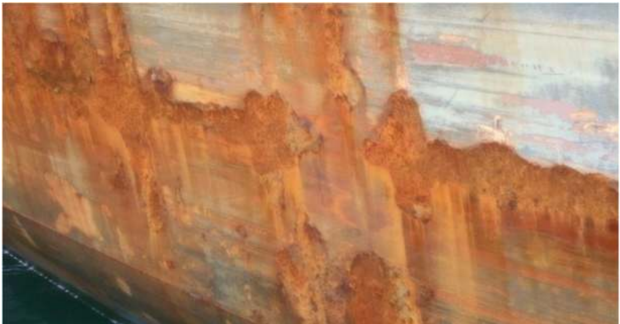
Corroded and wasted Hull
