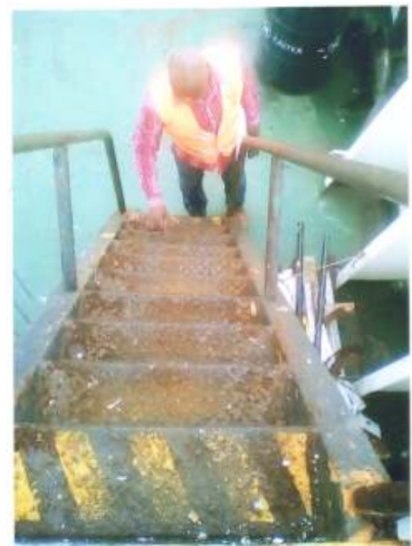
Corroded and wasted flight of steps
