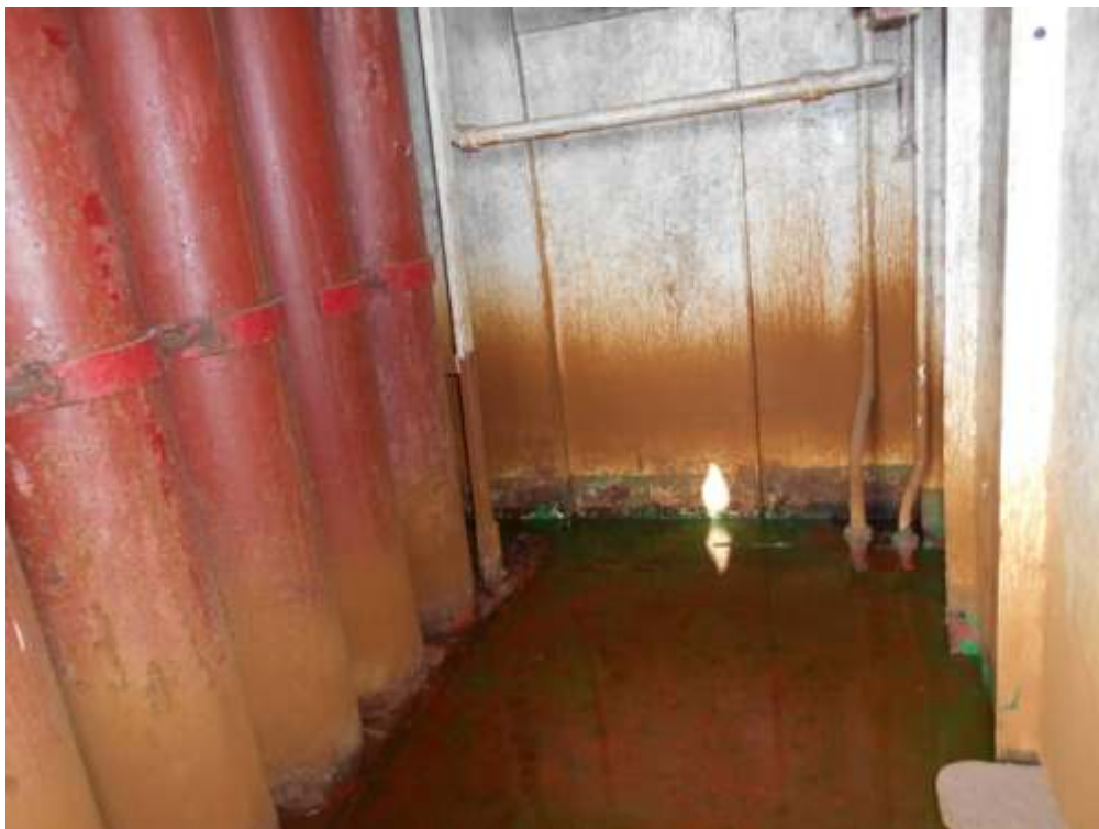
Corroded and Wasted Bulkhead
