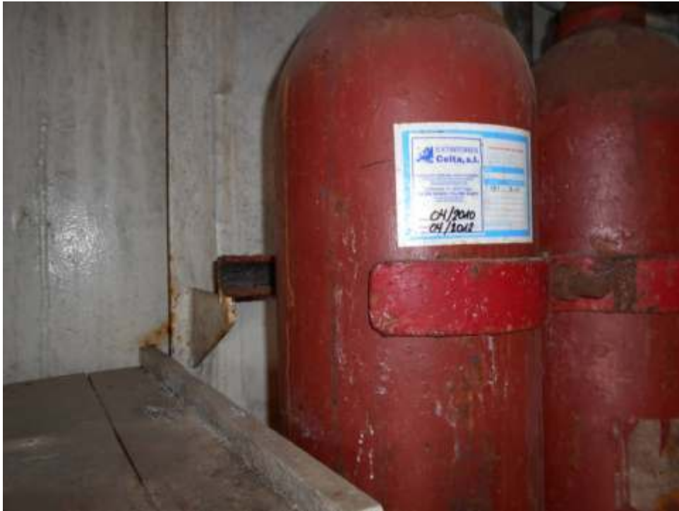
Expired Date on CO 2 Flooding Bottle
