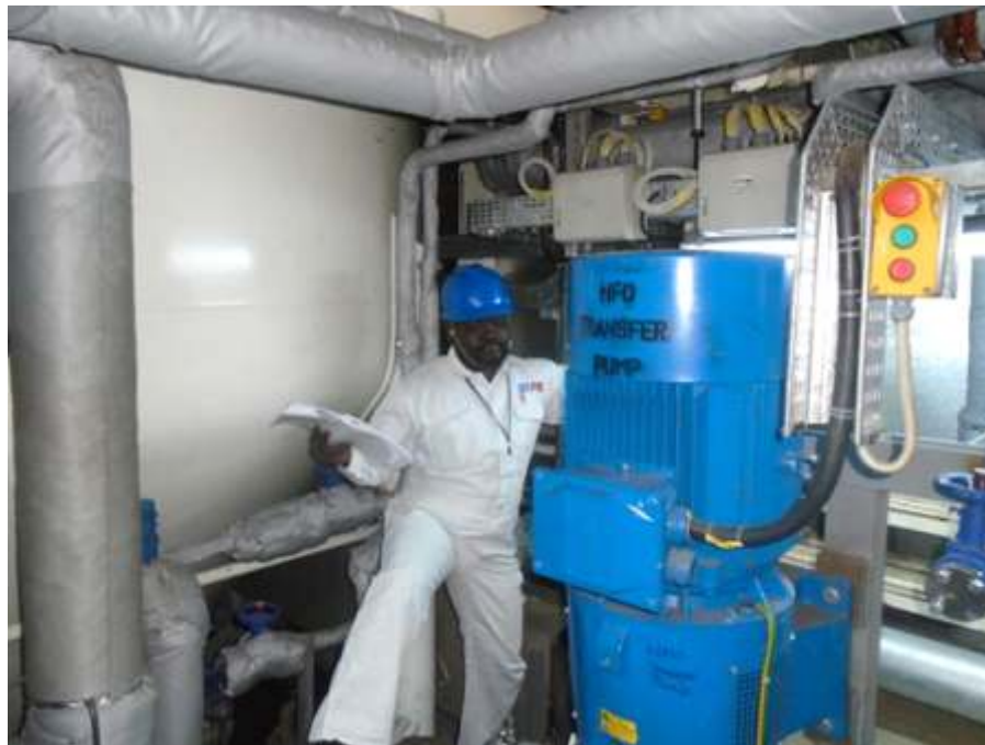
PSCO Inspecting HFO Transfer Pump
