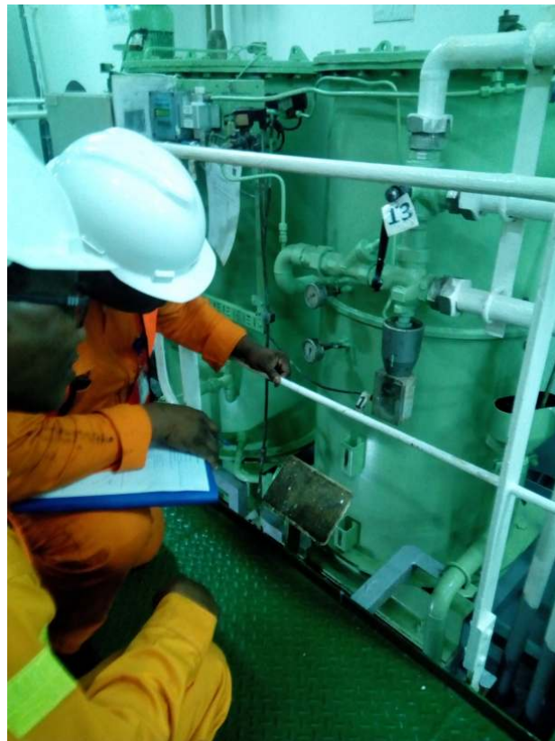
PSCOs Inspecting Oily Water Separator
