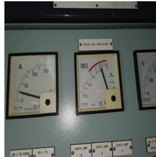
220 volts Insulation faulty
