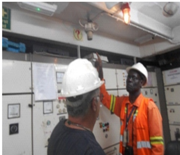
Senegalese PSCO inspecting the Smoke Detector Alarm in the Machine control room
