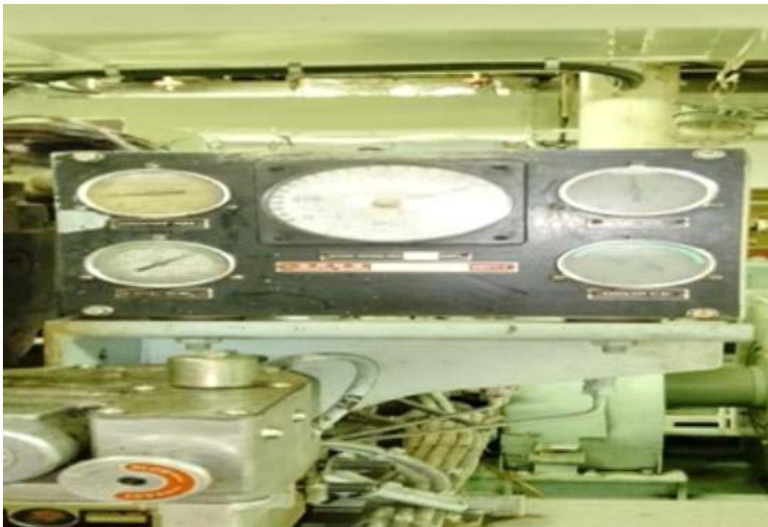
The Gauges that are difficult to read noted during inspection
