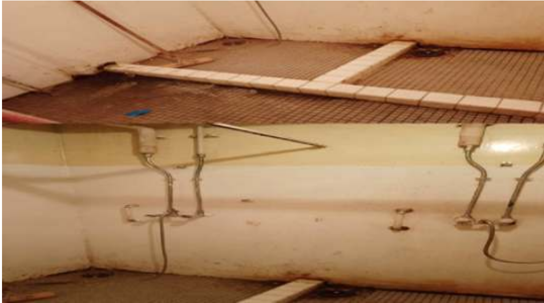
A dirty Shower-Room with damaged Shower Pipes observed during an inspection
