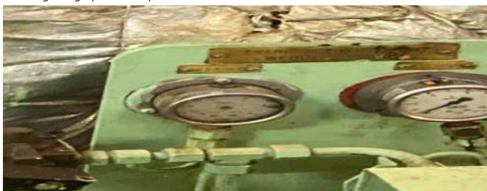
A Gauge with the Pointer Missing
