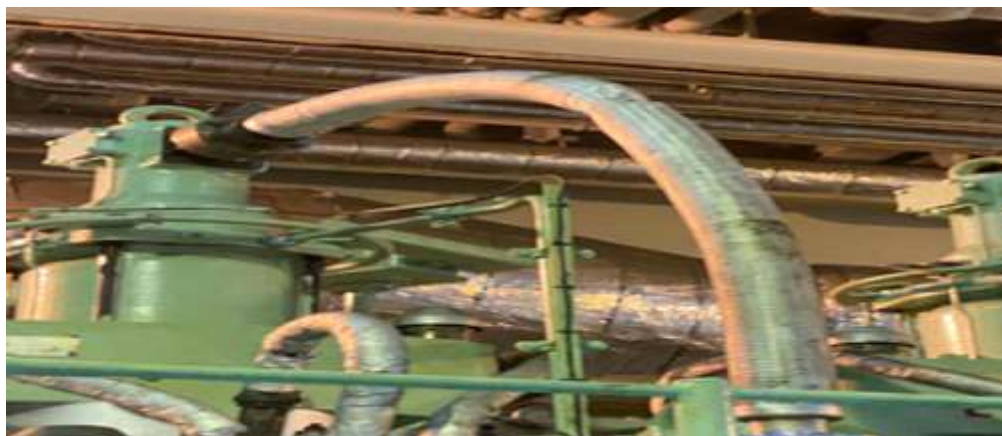
A damaged high-pressure Pipe Jacket
