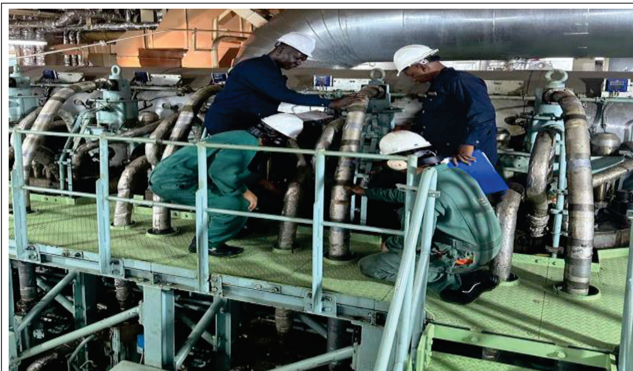
PSCOs Inspecting the Main Propulsion Engine Cylinder Head OCNEP inspectent la culasse du moteur de propulsion principal
